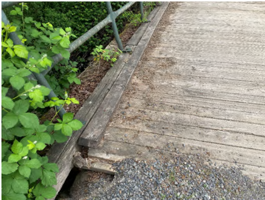
Photo 6 – Gordy Jolma No 10 Approach sloughing and hole at southwest corner
