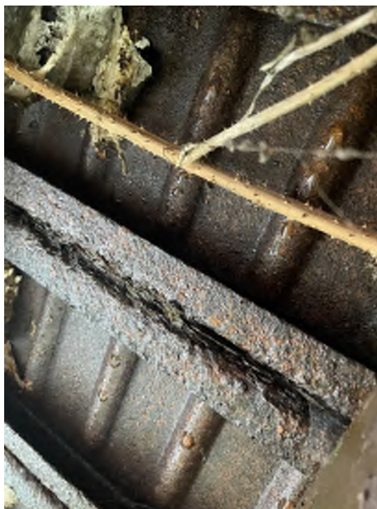
Photo 5 – Gordy Jolma No 1 Severe corrosion on deck plate and deck ribs.
