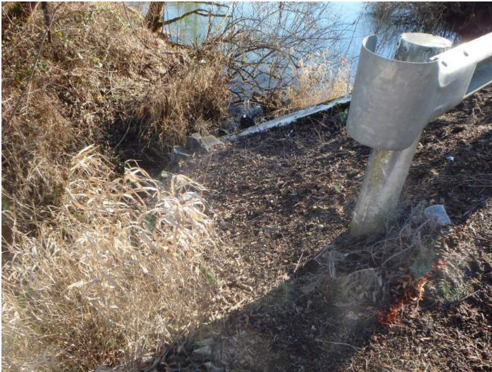
Photo 6: Smith Bridge – roadside ditch outlet to stream
