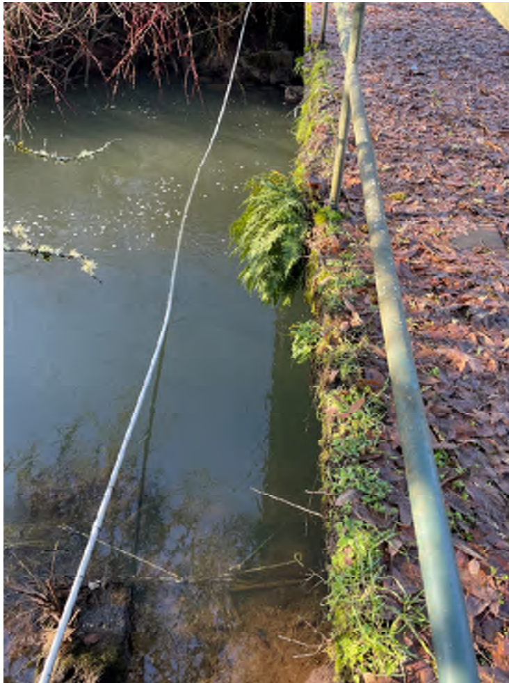
Photo 3 – Gordy Jolma No 3 view of failed 2” conduit in the stream.
