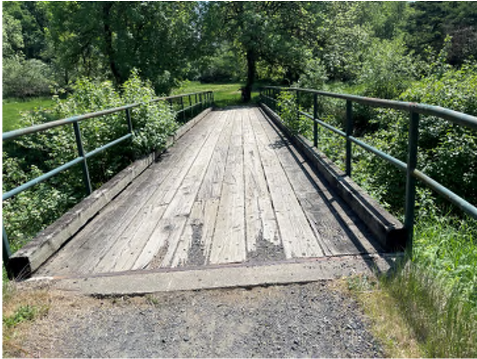
Photo 5 – Gordy Jolma No 7 Erosion and drop off at west abutment.
