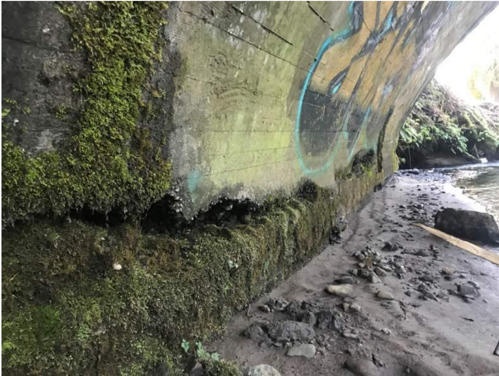
Photo 3: Salmon Creek Bridge – Concrete spalling
