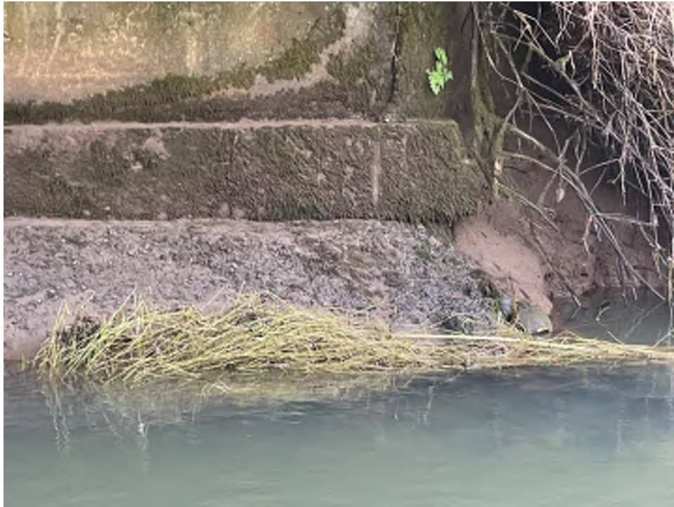
Photo 4 – Gordy Jolma No 9 Abutment Scour
