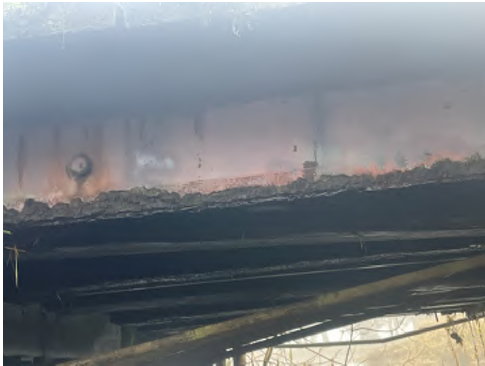
Photo 3 – Gordy Jolma No 10 Severe railcar corrosion and section loss and loose tie rods
