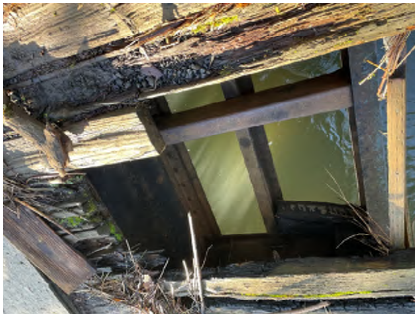
Photo 3 – Gordy Jolma No 4 Hole in Deck due to timber plank failure.
