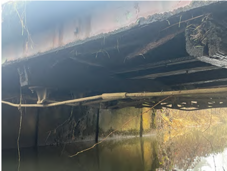
Photo 4 – Gordy Jolma No 10 Rotten timber floorbeams and loose tie rods
