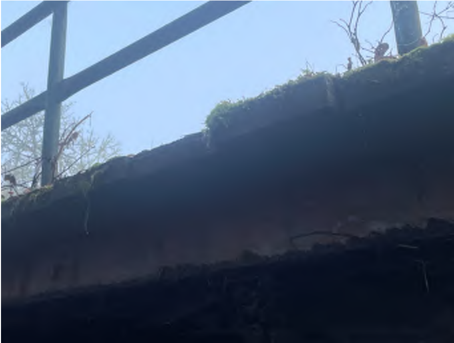
Photo 7 – Gordy Jolma No 10 Railcar steel section loss and timber deck rot and decay
