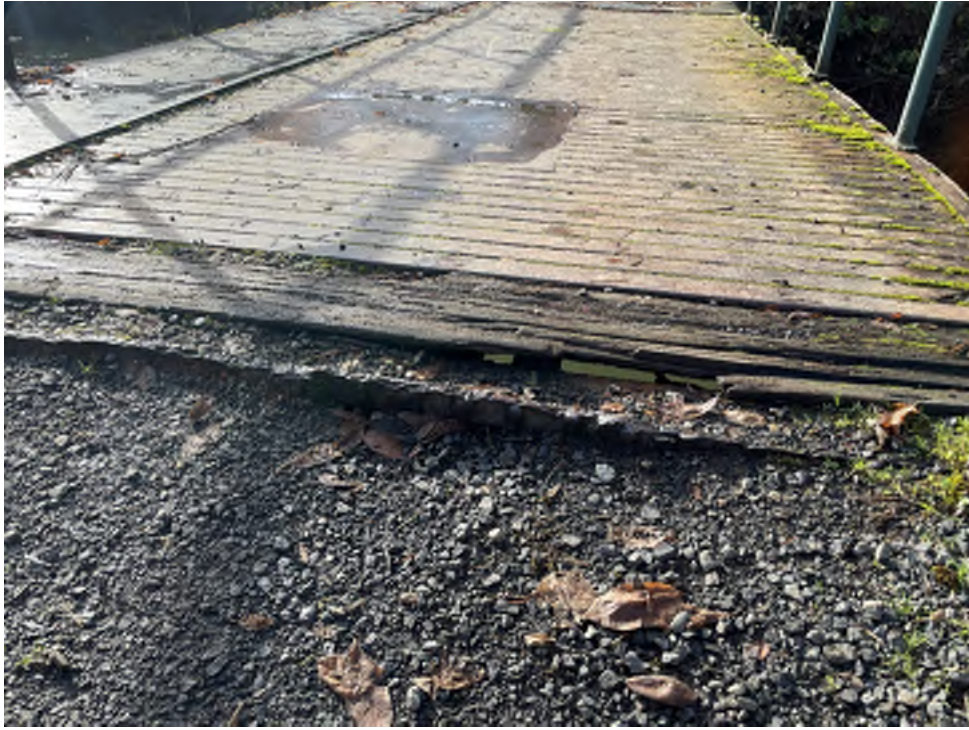
Photo 5 – Gordy Jolma No 6 Corrosion/damage on steel deck plate and erosion and drop off at abutment.
