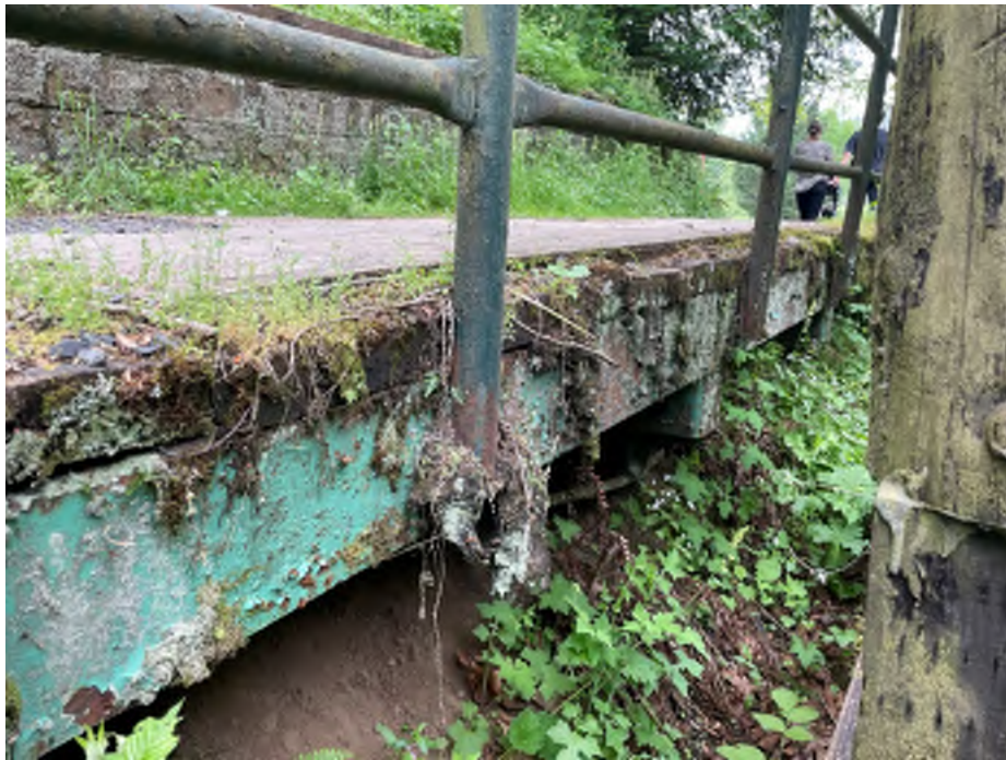
Photo 4 – Gordy Jolma No 11 Side Beam corrosion and loose tie rod.
