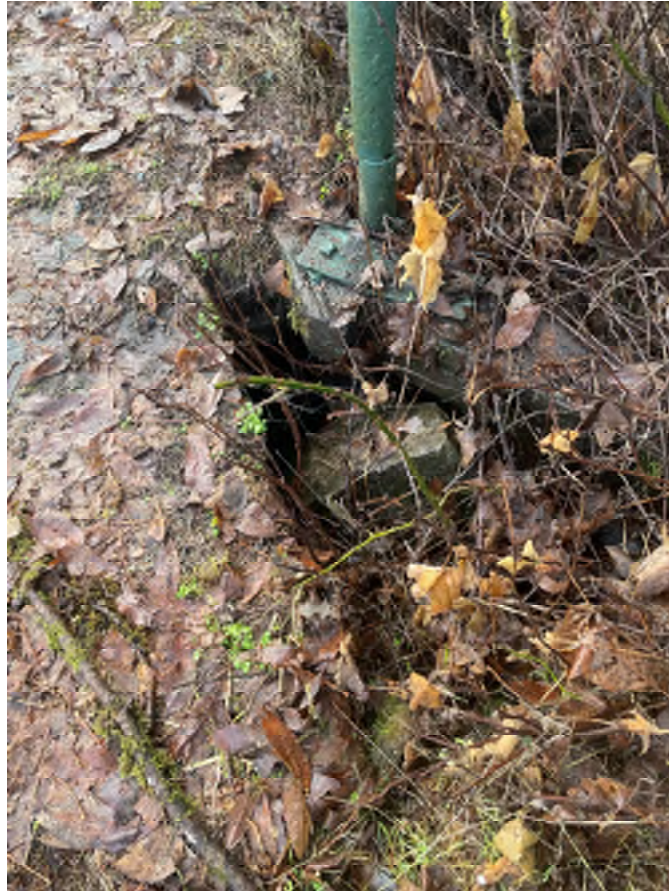
Photo 5 – Gordy Jolma No 10 Approach sloughing and hole at northwest corner
