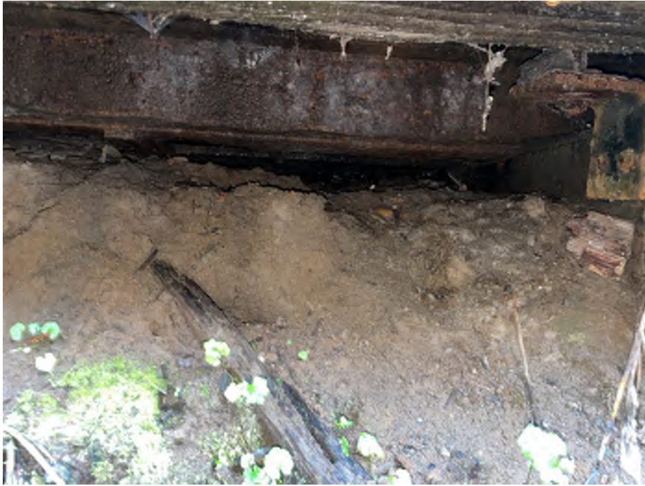
Photo 5 – Gordy Jolma No 11 Interior beam severe corrosion, pitting and loss of section.
