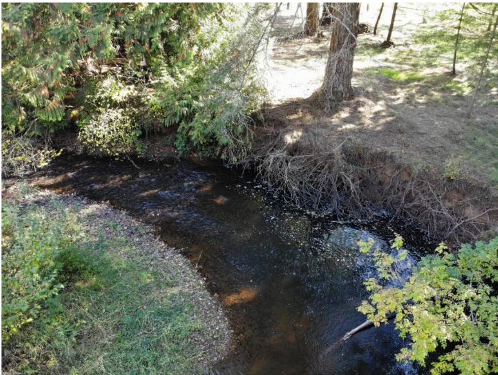
Photo 4: Smith Bridge - bank erosion downstream
