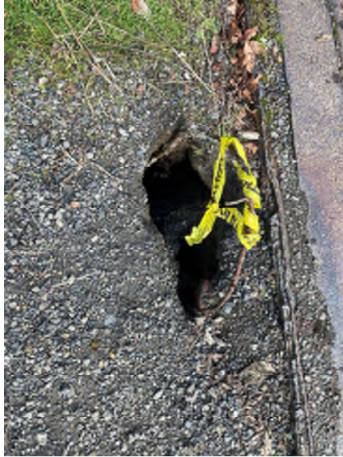
Photo 7 – Gordy Jolma No 9 Approach settlement and hole at north end, tripping hazard
