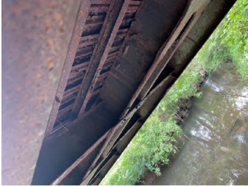
Photo 3 – Gordy Jolma No 8 Severe Corrosion and loss of section steel stringers and bottom of deck surface, crevice corrosion, and fatigue-prone details.
