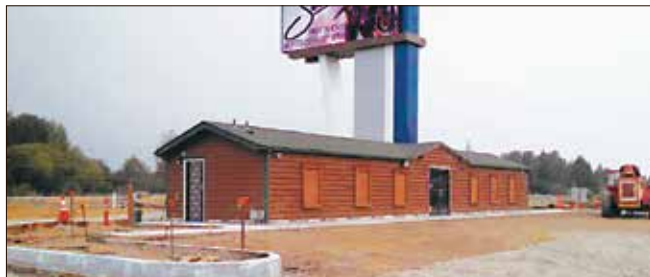
Economic development from the foundation up! The Cowlitz Tobacco Outlet in progress.
