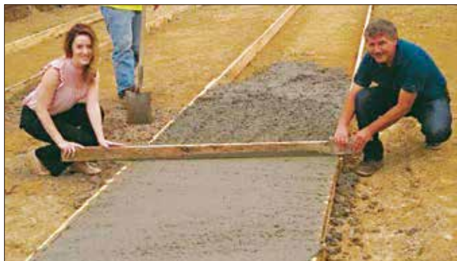
Economic Development committee members Whitney (Devlin) Mosback and Tim Van Mechelen leveling the concrete on a foundation footing for the Cowlitz Tobacco Outlet.
