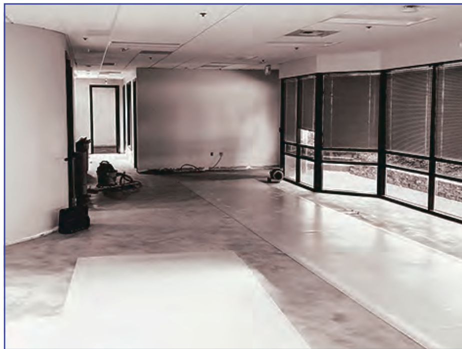
Work progress on the new MAT office in suite 102 of the new tribal building in Tukwilla.
