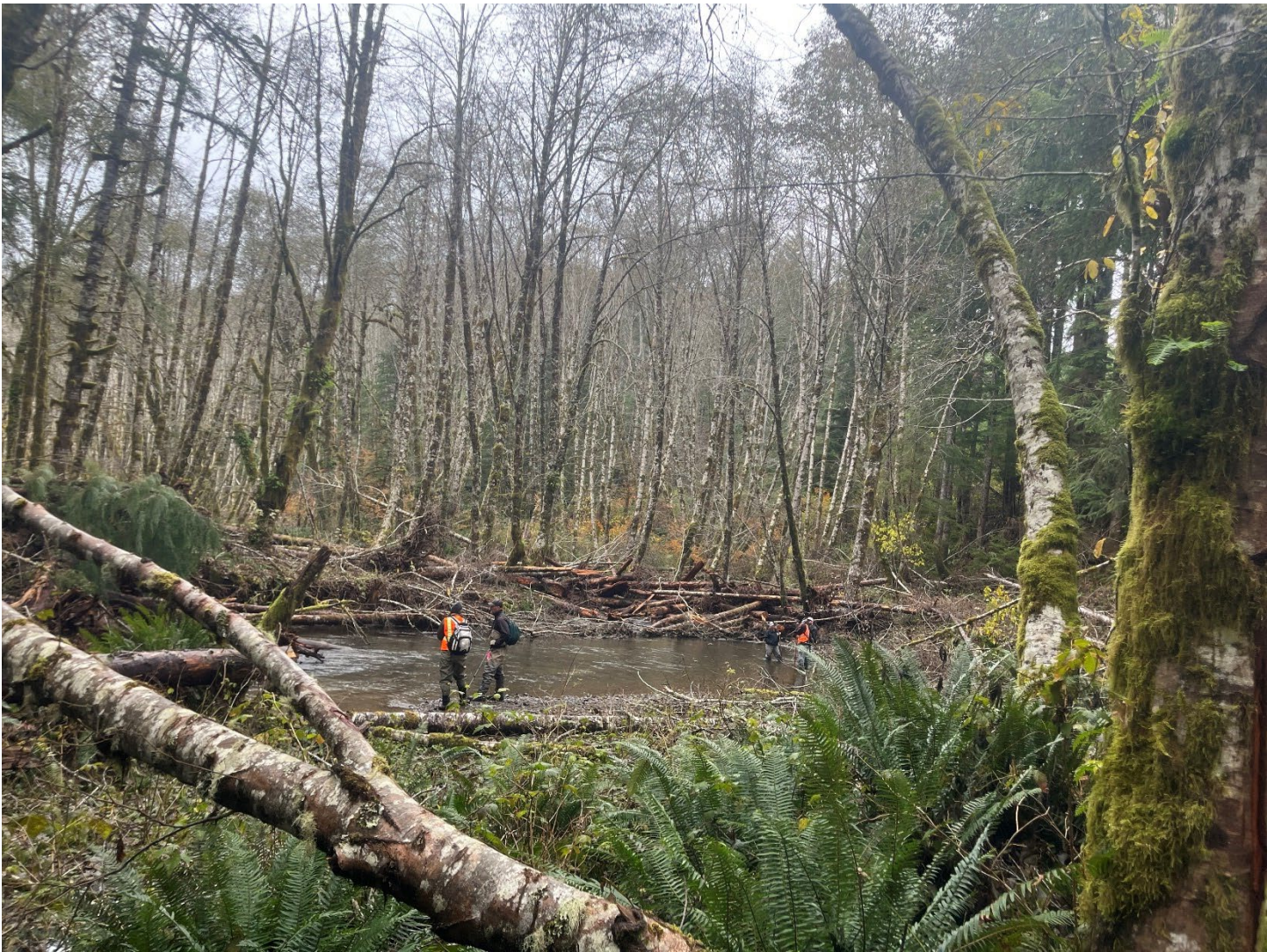
Figure 1: Mitchell Creek project site from the Lower East Fork Grays Restoration project demonstrating conditions for thinning, brushing and planting in this area. Note the presence of engineered log jam in the channel.
